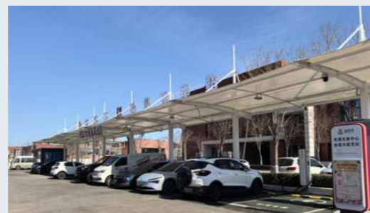
Beitang Culture and Sports Center Fully Liquid-Cooled Ultra-Fast Charging Station
